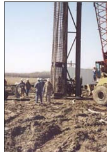
O-cells can be Placed at two Levels in the Shaft to Isolate Distinct Shaft Elements
